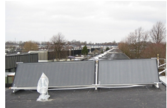
Solar panels - roof mounted. Photo: NOVA5
