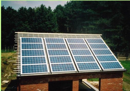
Photovoltaic panels on the roof of the garage
