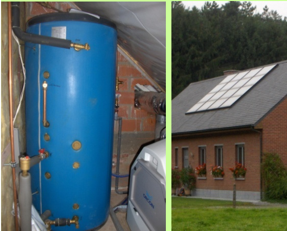
The buffer tank, and the solar collectors installed on the roof
