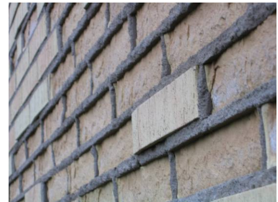
Worn out masonry facade
