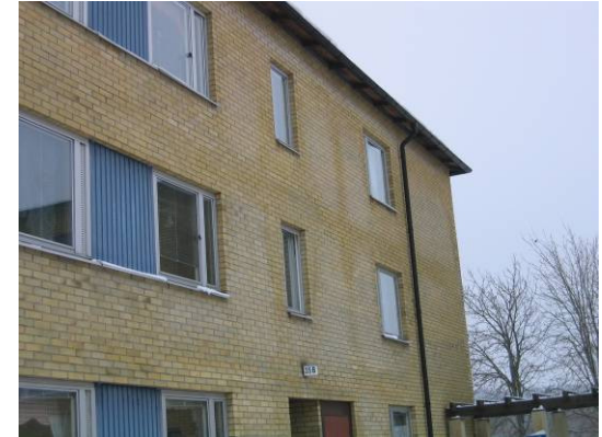
Existing facade with thermal bridges
