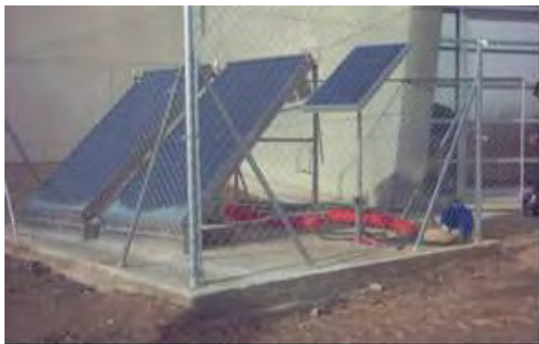
Figure 2-2 Solar thermal collectors from Takama.
