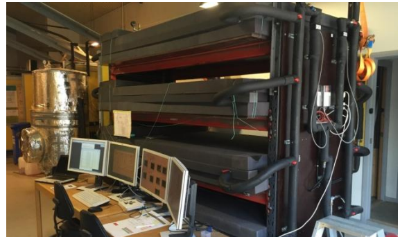
Figure 19: PCM heat storage with four modules for the demonstration system.
