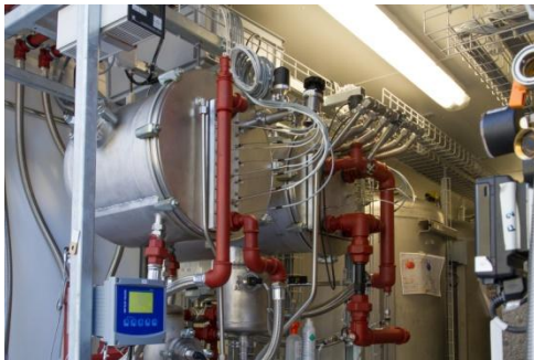
Figure 5: Picture of the demonstrator heat and mass exchanger connected to the storage tanks.
