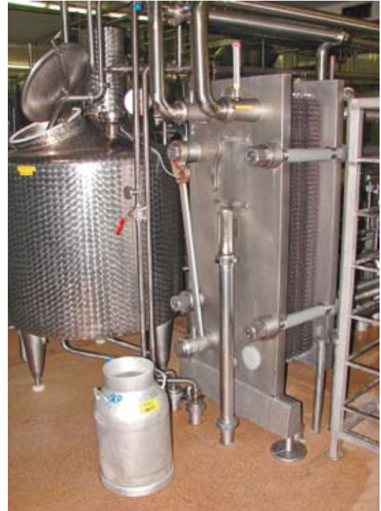
Installed heat exchanger in an Austrian dairy (Source: JOANNEUM RESEARCH, Austria)
