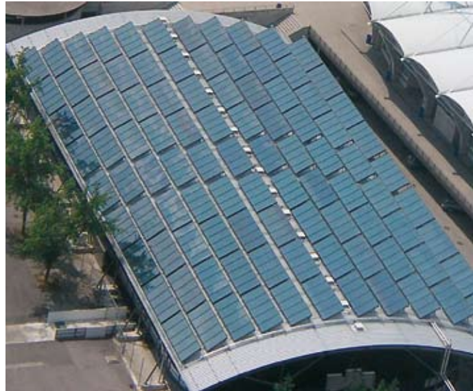
Solar thermal plant, football stadium “UPC-Arena” in Graz, Austria (Source: SOLID, Austria)
