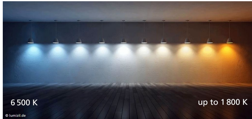
Figure 6 | “Tunable white” solutions make it possible to adjust the colour temperature e.g., in the course of the day following the daylight. [© lumizil.de, Fraunhofer IBP]
