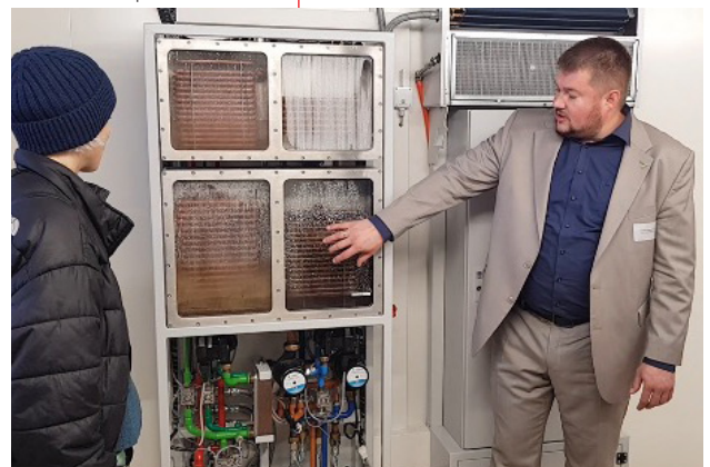
▲ The Green Chiller Association offered a tour around a mobile sorption classroom. The completely open absorption cooling system makes it possible to explain the technology clearly and illustrate various operating states. Christian Kemmerzell, Managing Director of EAW Energieanlagenbau, demonstrates the unique system. (Photo: Bärbel Epp)
