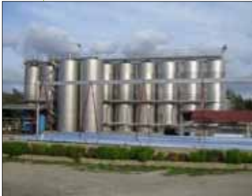
The solar cooling system installed at this Tunisian winery was monitored by Task 38 experts and received the Energy Globe Award Tunisia 2009.
