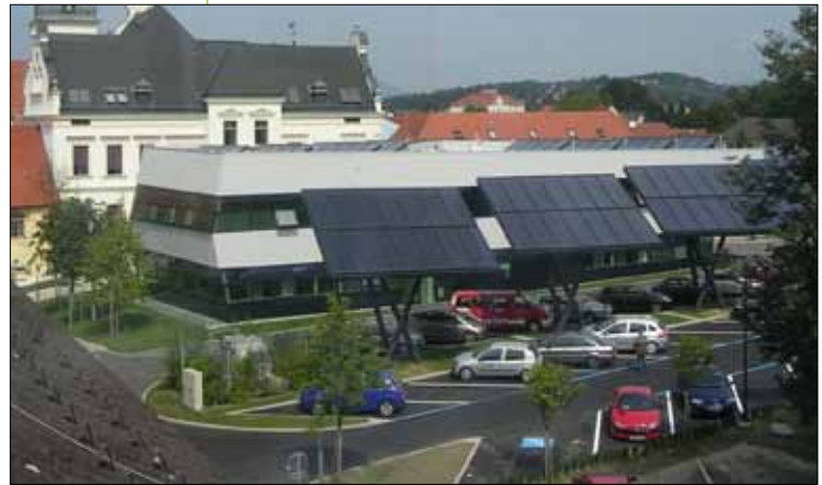
▲ Figure 2. Solar heating and cooling installation at the Town Hall Gleisdorf, Austria (304 m 2 flat plate collectors connected to 35 kW Yazaki chiller WFC 10 and a desiccant evaporative cooling system). (Source: AEE INTEC)
