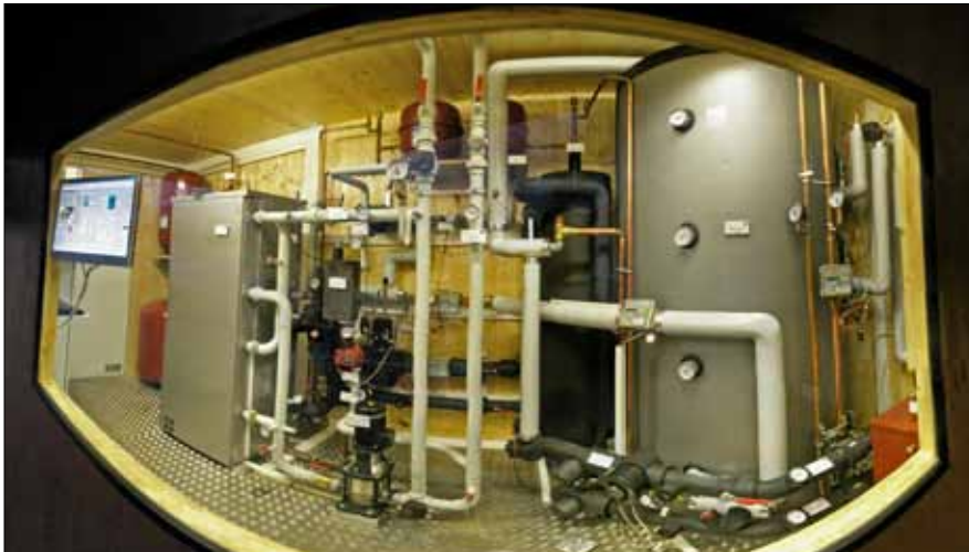
◀ Figure 3. Indoor components of the solar cooling installation at the office building of the Company SOLID in Graz, Austria (17.5 kW Yazaki chiller WFC 5). (Source: SOLID)
