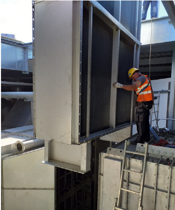
Installation of the air/water exchanger (10t) in the Lactalis spray drying tower (source: Newheat)
